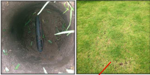
Figs 6 & 7. Exposed irrigation pipe (left) and extra growth coinciding with emitters (right).
